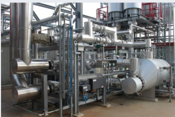
Hot Oil / Water Transfer
